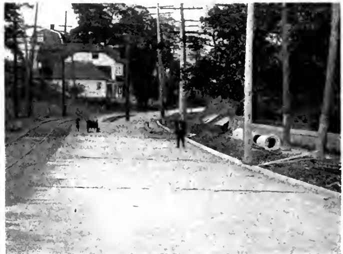
Fig. 5—The commission reduced the bank and made a simple curve with clear vision.
